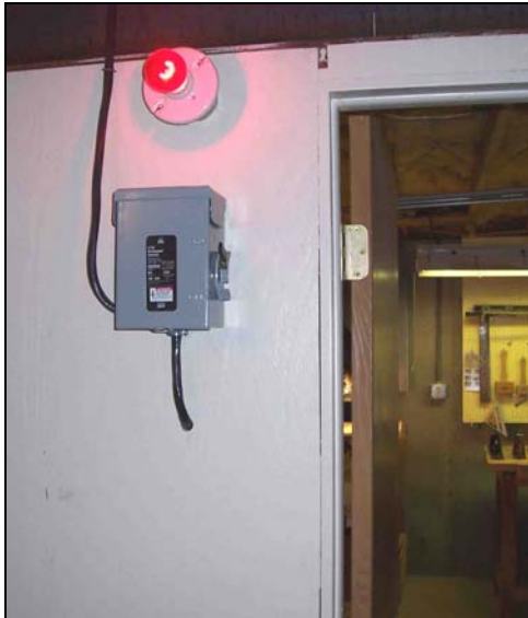
Master power cutoff – a good idea for everyone from a safety and fire standpoint.
