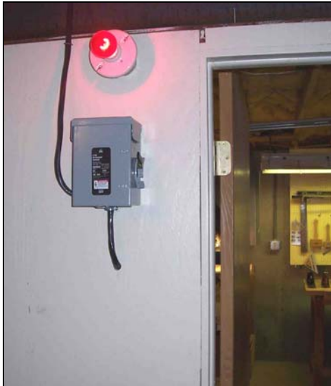
Master power cutoff – a good idea for everyone from a safety and fire standpoint.
