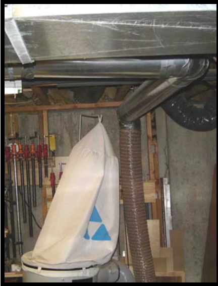
Allen uses large main ducts running off of his collector to reduce loss in his system
