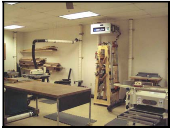
Another view of duct port wall, wood storage, clamp rack. Delta air cleaner cleans air and also helps circulate heat.
