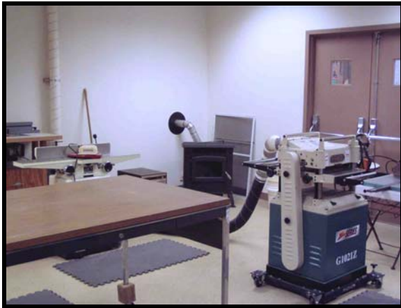
Looking back at the doors. Note the blocks raising the outfeed table. Pellet stove provides heat. Dust collection ducts on the one wall. Jointer and planer, largest chip generators, placed closest to dust collector. The planer is an 18" unit and the jointer a 6" model. A dehumidifier is installed in the shop.
